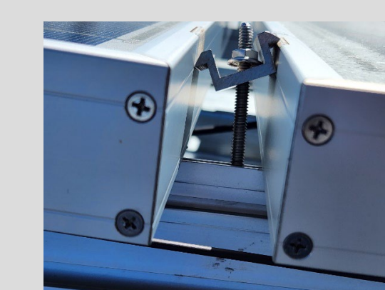
Top-clamp fails in high wind
