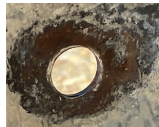
Image 3: Example of Fretting Wear Of G90 Purlin at Joint Interface Due to Repeated Joint Slip
